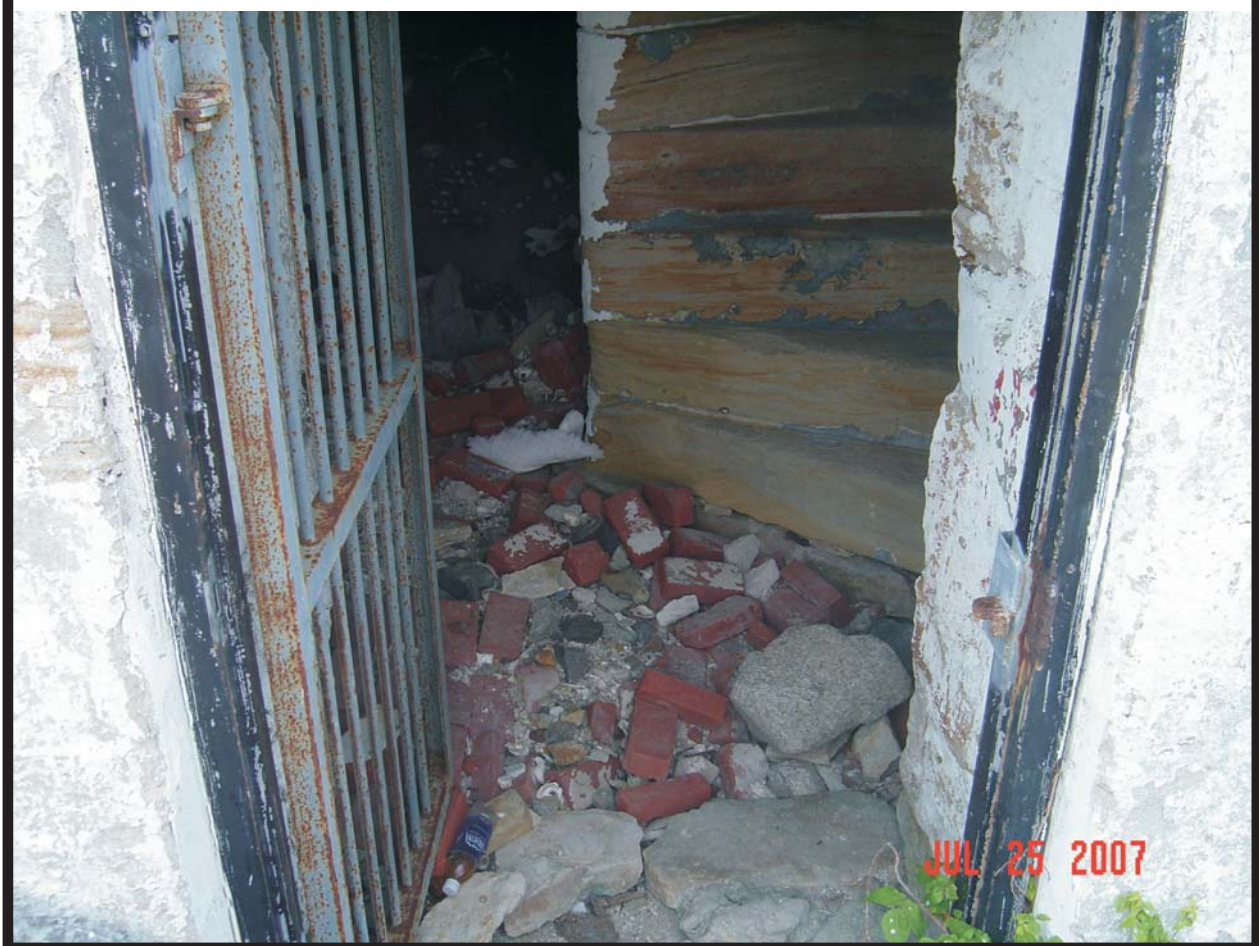
Figure 14. The door to the lighthouse is open exposing the interior to the elements and wildlife.
