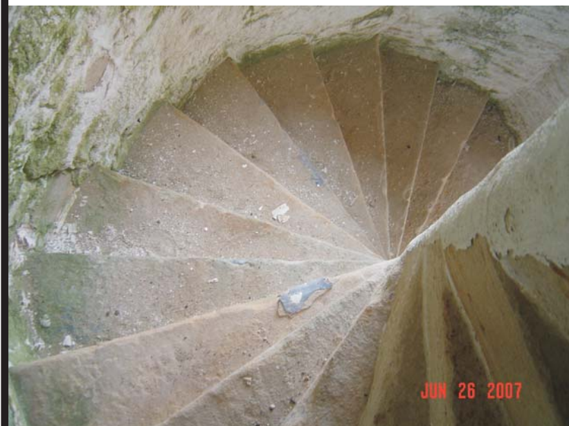
Figure 15. Photos depicting the present state of the interior of the lighthouse. The sandstone steps are exposed to the elements and eroding. The upper level platform is only being held up by a 2x4.
