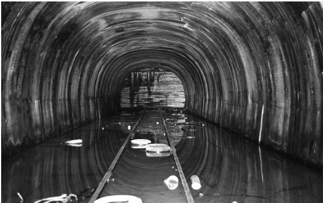
Figure 15 - An image of the flooded eastern entrance to the Church Hill Tunnel (Public domain, by Wikipedia user Jkmscott)
