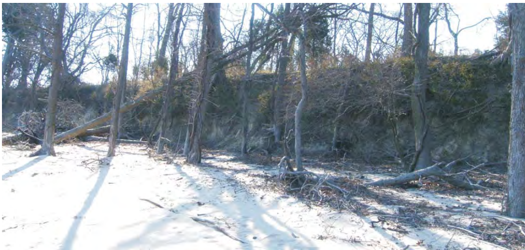
5. Bank erosion in front of the pond.
