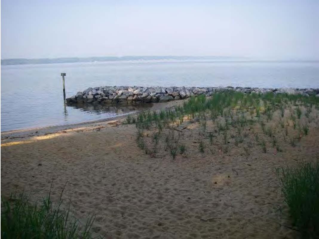
Figure 3. New breakwater constructed at J36. For 2010, the seine haul location was moved approximately 50m downstream to accommodate for the breakwater placed directly over the historic index station.
