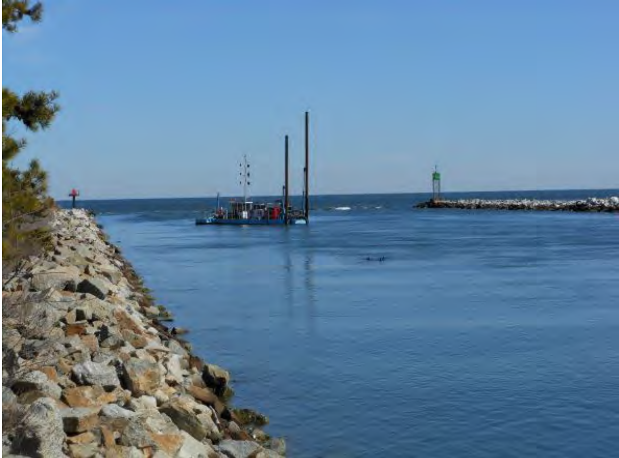
Photo 1. Dredging of the Little Wicomico River Federal Navigation Channel in 2010. Photo courtesy of the U.S. Army Corps of Engineers, Baltimore District.
