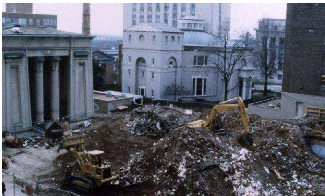
Figure 1: Construction of MCV's Kontos Medical Sciences Building in 1994. The building is located at 1217 E Marshall St, Richmond, VA 23298
