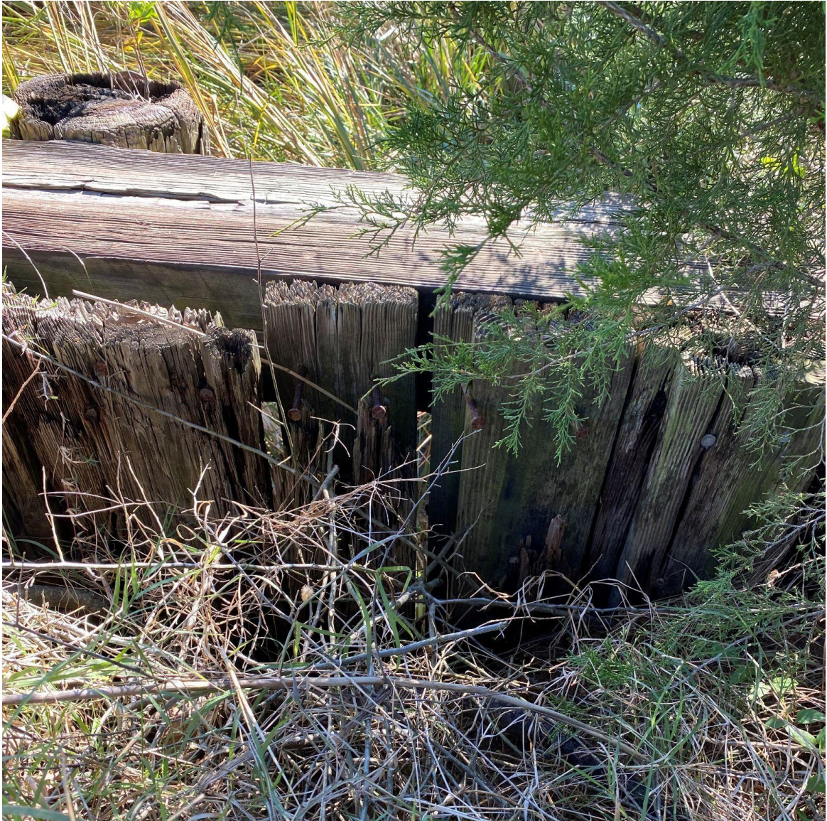
Figure 13: Pit that formed behind the dilapidated bulkhead at Site 2. K. Grigsby, 2022.
