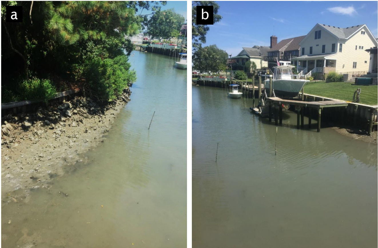
Figure 4. Photos of Section C showing: a) the seawall fronted by riprap that makes up most of the northern side and b) the seawall without riprap on the southern side.
