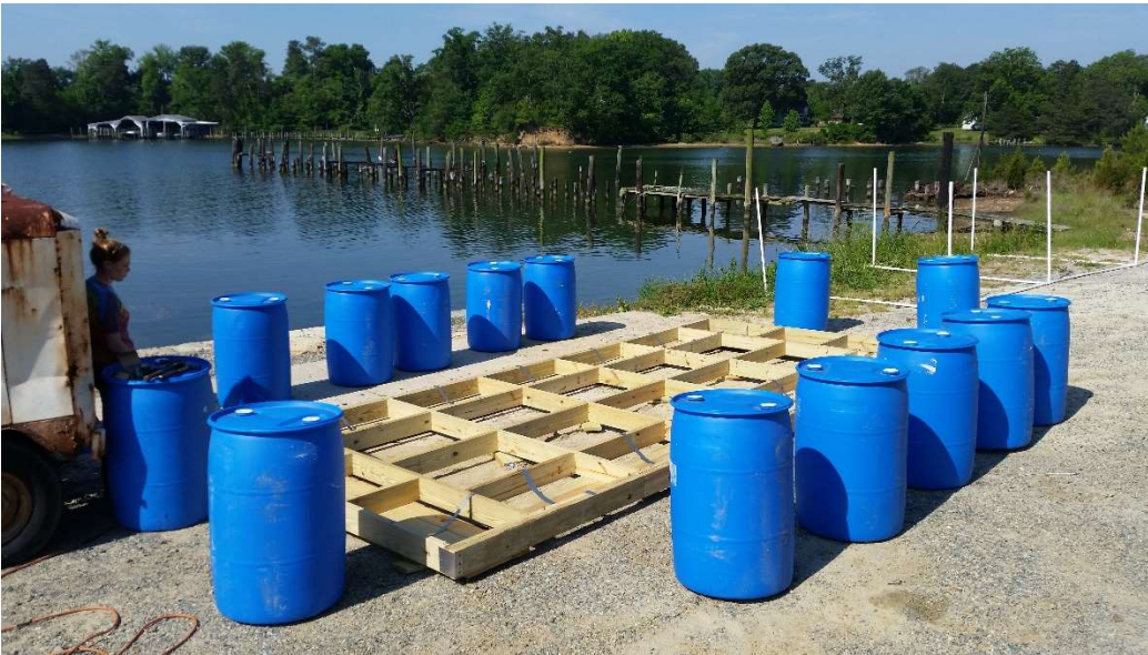
Barge has been flipped.
