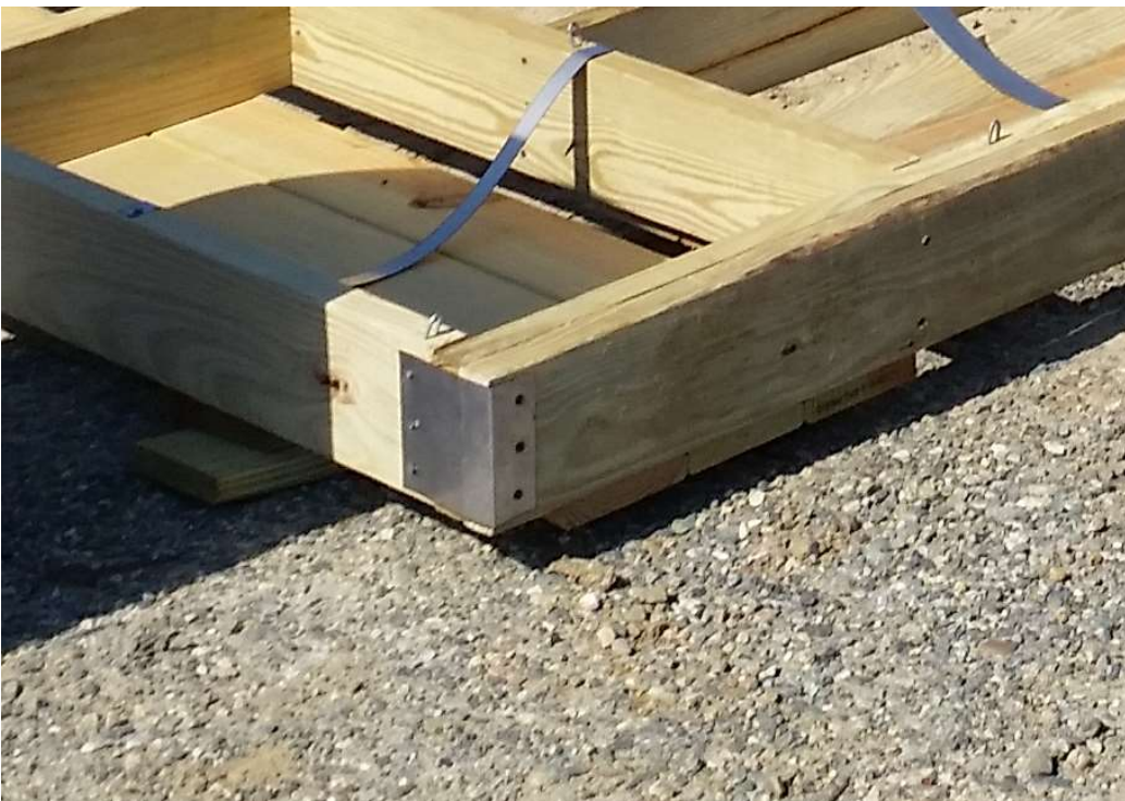
Caption: Again, note the barrel strap that will be on the top of the barrel and the metal plate around the corner. Both of these keep the stress of the weight from popping the screws.
