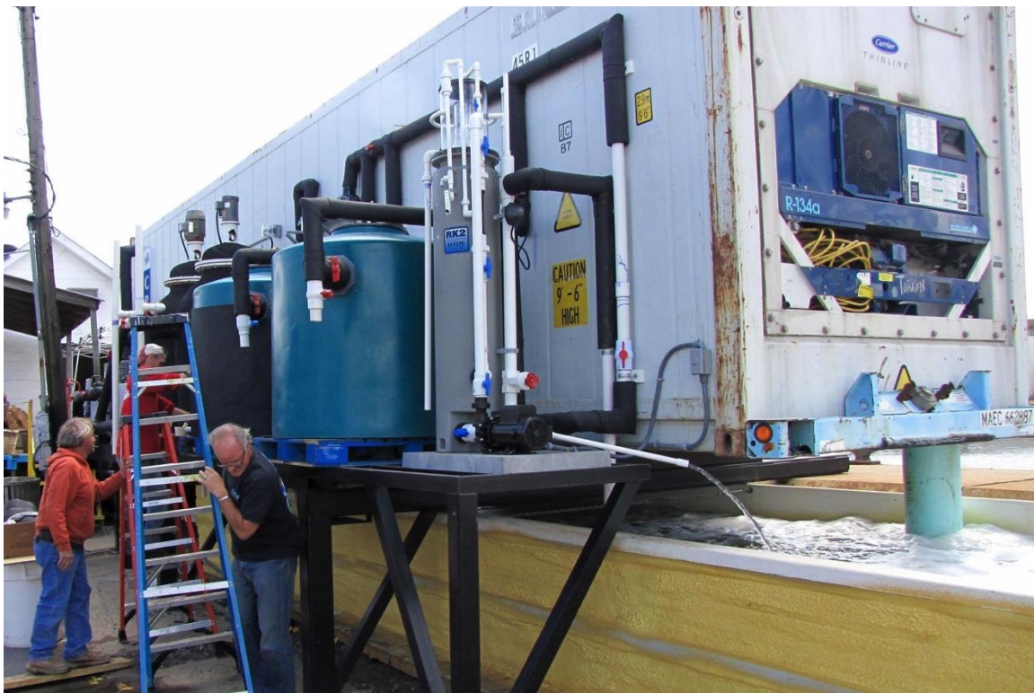
Construction of the large holding system in Newport News was almost complete when this photo was taken in April of 2015.
