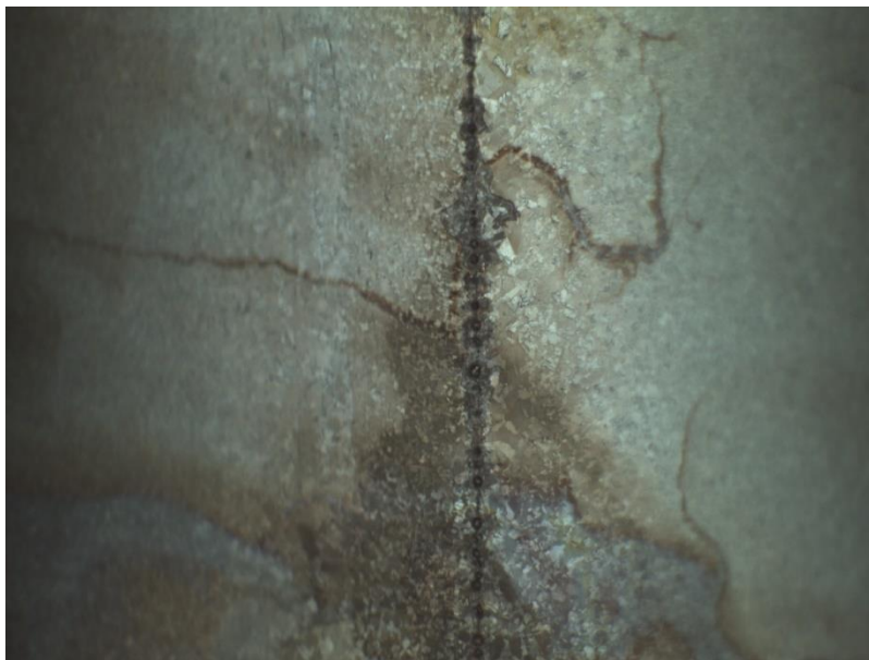
Figure 6.8: Internal inspection photo of Cu cavity after EP showcasing equator weld crack and chemical trapping.
